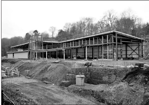
The SVR's new 'Engine House' is rapidly taking shape at Highley as seen 23rd February 2007. 7325 should be in residence later this year.
